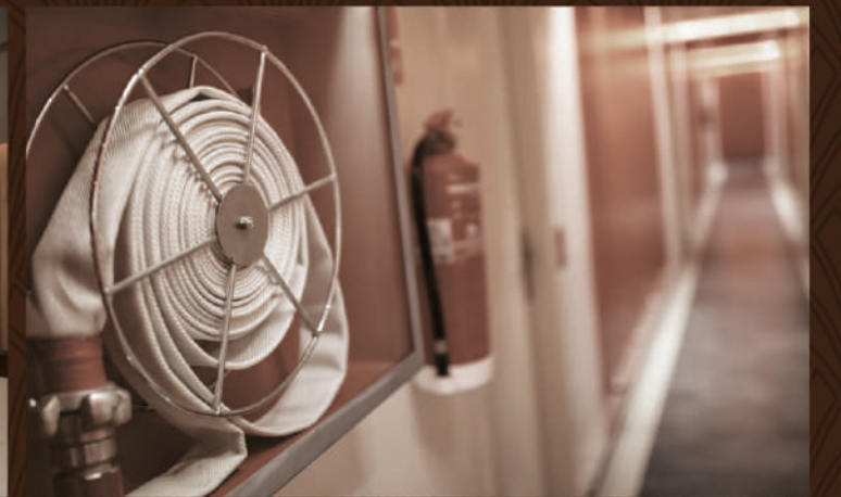
Fire Safety System
