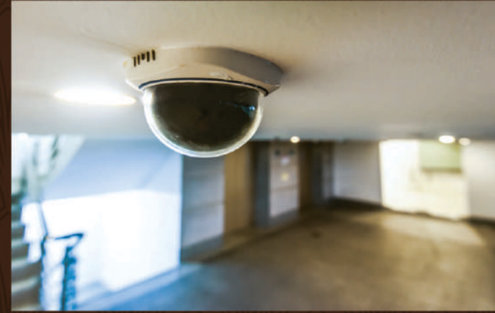
CCTV and Manned Surveillance System
